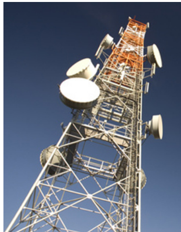
Figure 1.2: Base station antenna(Label Italy | Log 8 Elements FM Antenna Systems | FM Systems).
